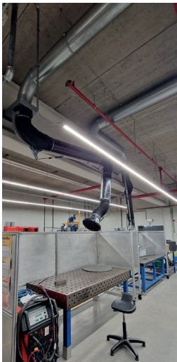
Extraction arms linked to a central filtration unit.
